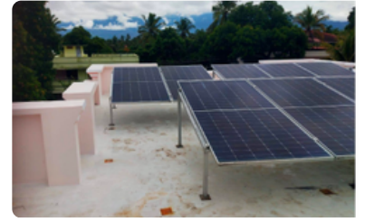
MANAF PALLIPURAM POWERS UP SUSTAINABLY WITH 12 KWP SOLAR
