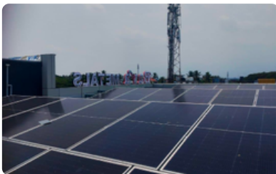
BALA CINEMAS GOES SOLAR WITH 73.85 KWP PLANT!
