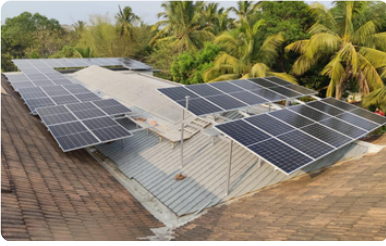
MOTHILAL GOEL GOES GREEN WITH 30 KWP SOLAR PLANT
