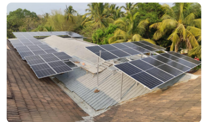
PYARELAL FOAMS TAKES A SUSTAINABLE STEP WITH 11 KWP SOLAR PLANT!
